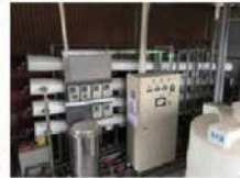
Water circulation system in Suzhou factory
